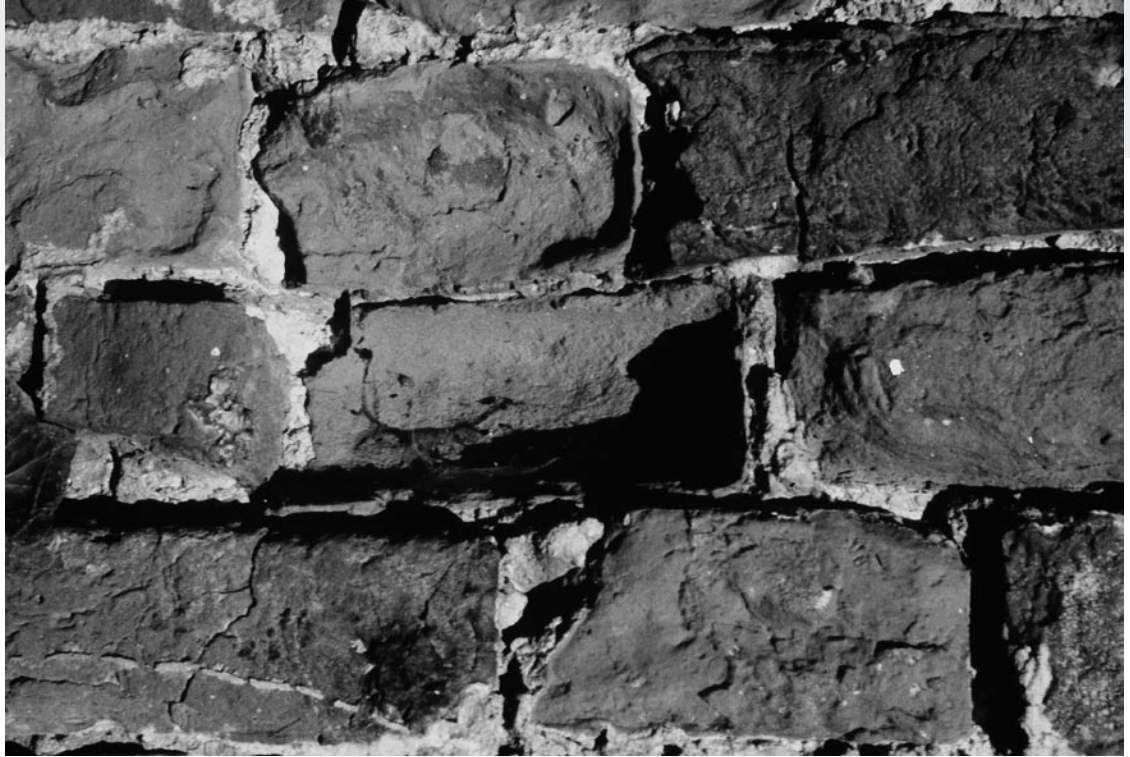
Fig. 3: Freeze / Thaw damage
